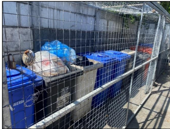
Figure 10. Bin cage at Forest Glade Retail Centre that requires modification.
